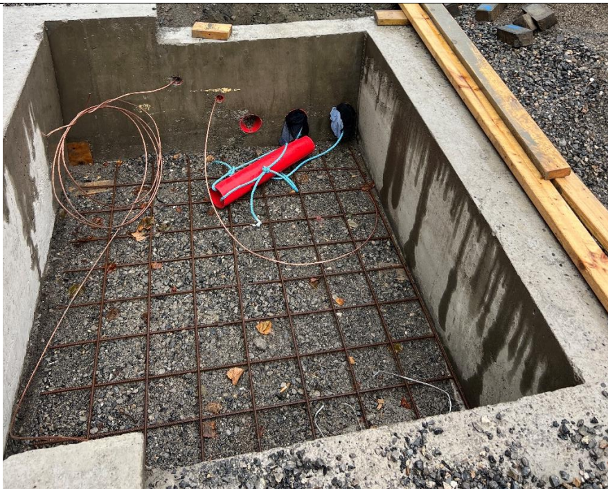
Date: 25 th Sept 2024 Substation Joint Pit – Earth Cable Installed and Ducts Proved.
