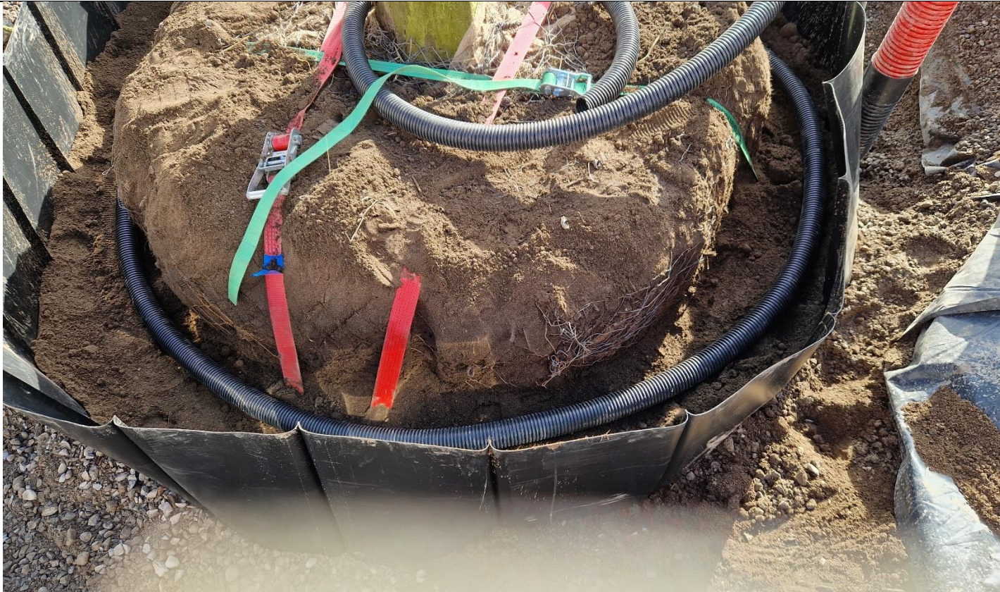
Date: 07 th Feb 2025 Tree Roots Drainage System
