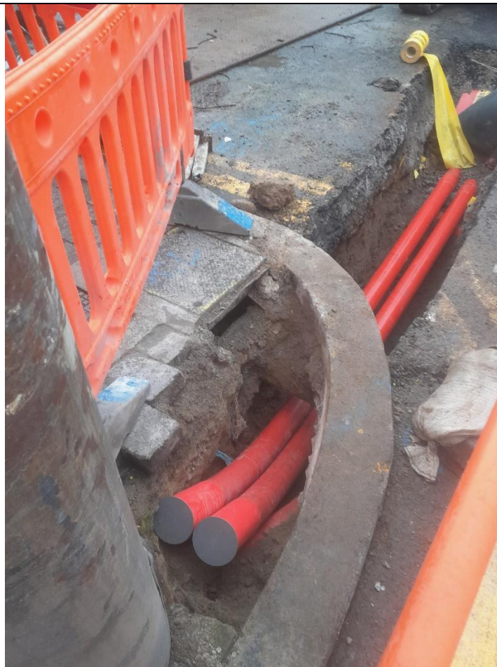
Date: 18 th December 2024 Installation of ESB Ducting to Pole on Leinster Road
